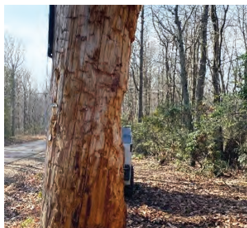
NOVEC needed to replace this pole after a bear did serious damage with its claws.
